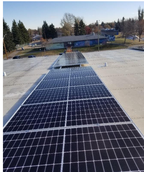
Solar panels were installed on the arena in 2021
